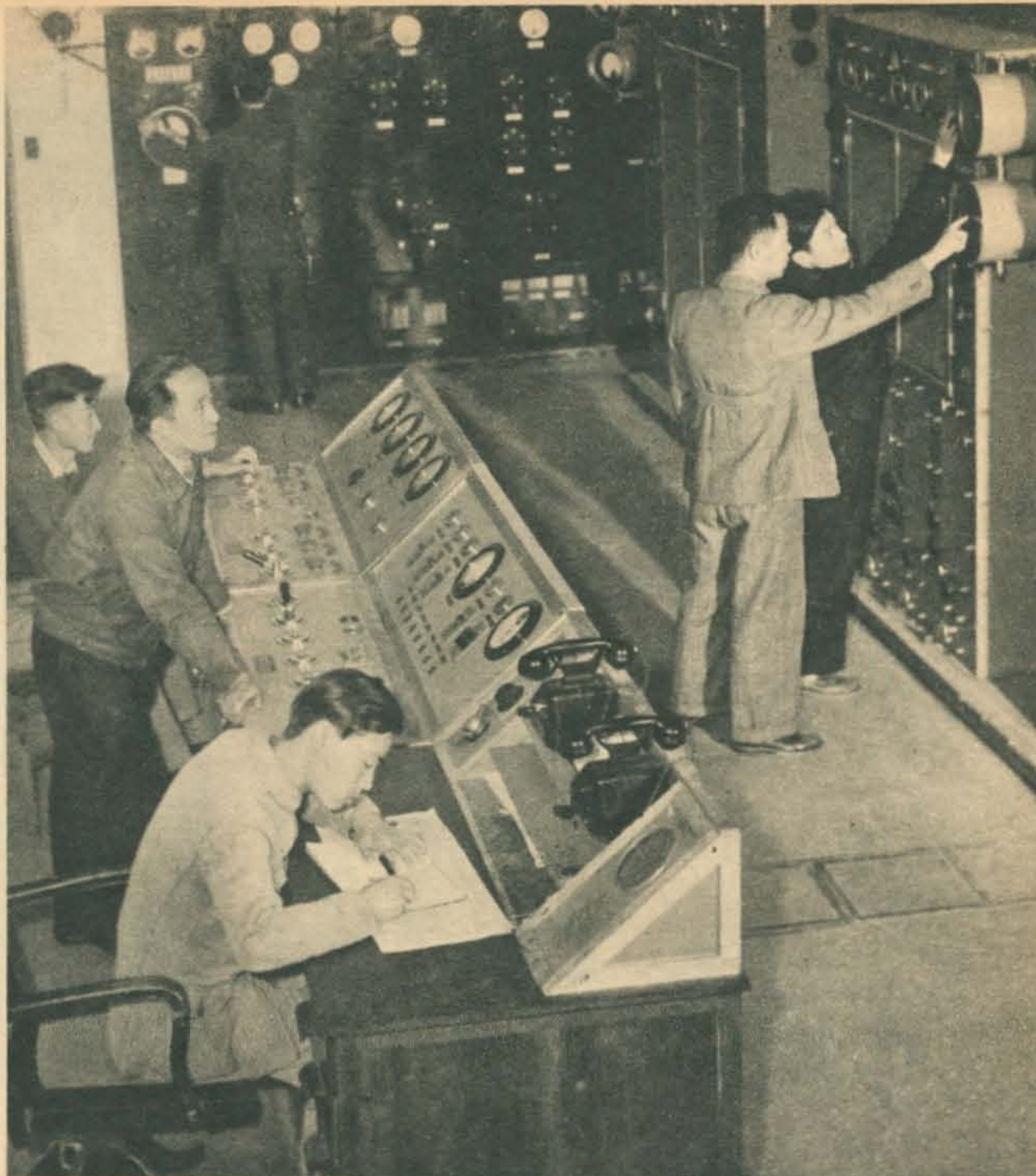
THE TRANSMITTER ROOM OF STATION XGOY IS LOCATED IN A CAVE NEAR CHUNGKING
