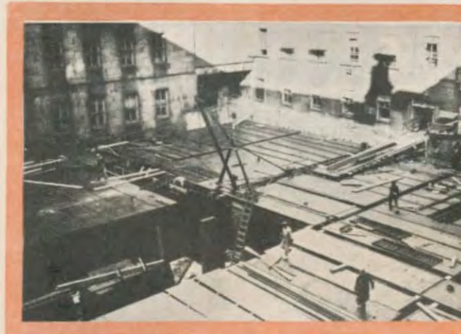
The new vault in course of building. It occupies an old courtyard of the Treasury building.
