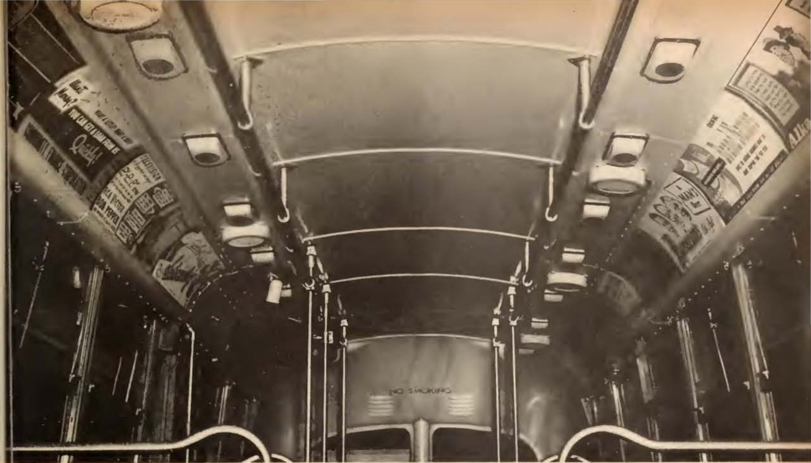
In a transiradio installation one speaker usually alternates between two lights to bring riders an equal volume of sound without blasting at any point
