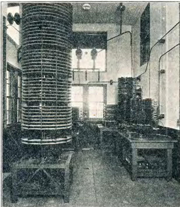
Tuning inductances, relays, and signal control apparatus of one of the six transmitters.
