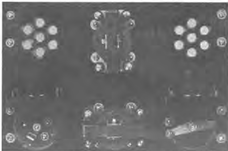
Rear View of Completed Amplifier Panel
