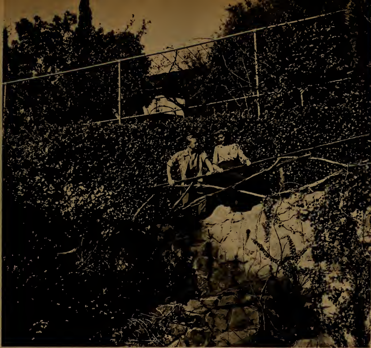
The remodeling of stable and guest house—and the moving of materials and furnishings—was even more of a problem than it sounds. Here's the hill down (and up) which all those materials, all that furniture, had to travel.
