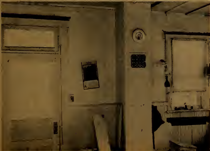
BEFORE: This dismal area of the kitchen was vacated by a big, black pot-bellied stove with coal bucket nearby.
