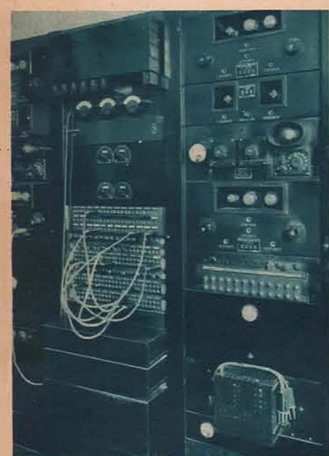
9 The cross-country telephone wires lead to switchboards (above) at stations on the net
