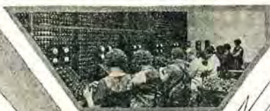
5000 telephone switch-board—operators testing Elkon rectifiers and the seasoning boards in the background.
