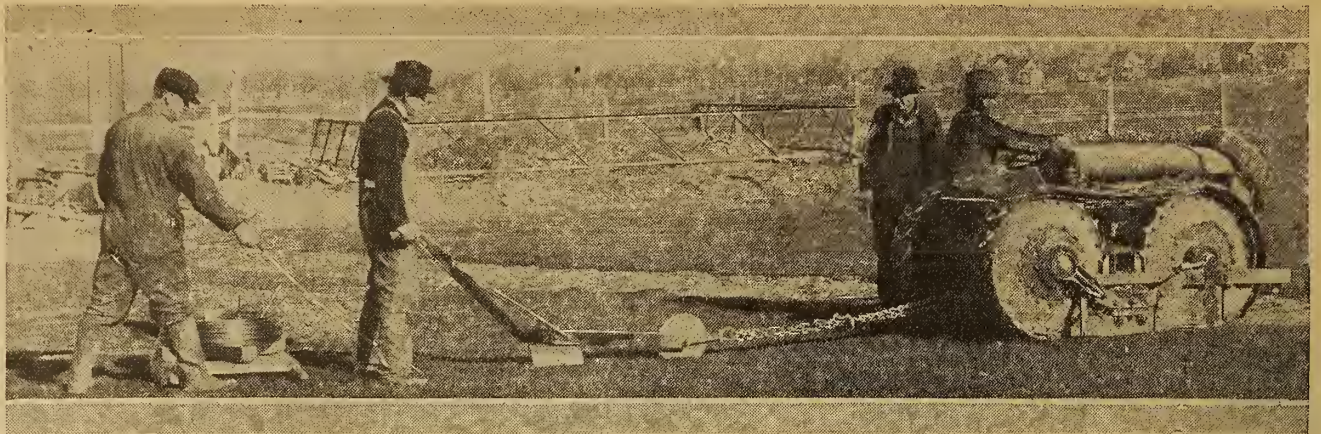
This is the way that Station WCBD, Zion, Illinois, is laying the ground wires for its new super power station. The wire is attached to the heel of the plow and follows in channel made by point. The wire is laid ten inches deep. A thin knife makes an incision, while the lawn remains undisturbed. Nine and one-half miles of wire are required.
