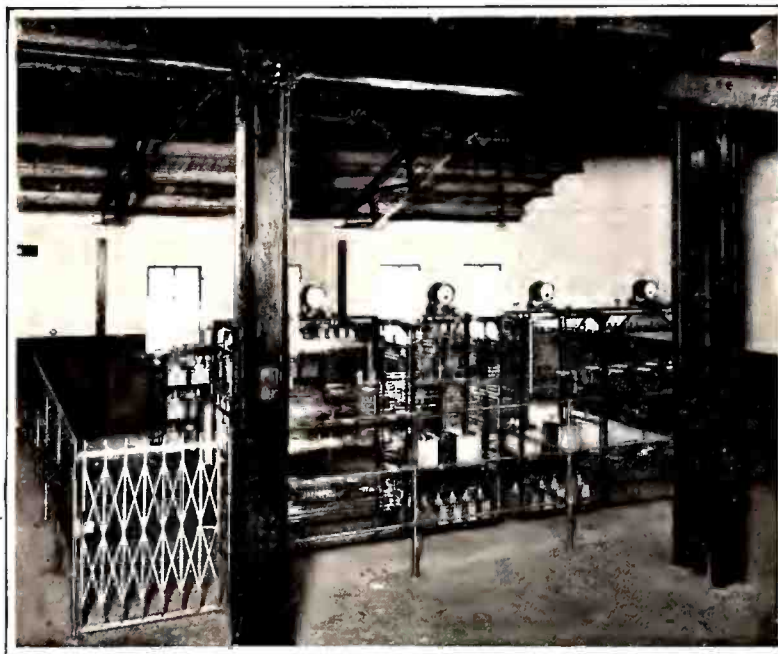
BEAM STATION EQUIPMENT
