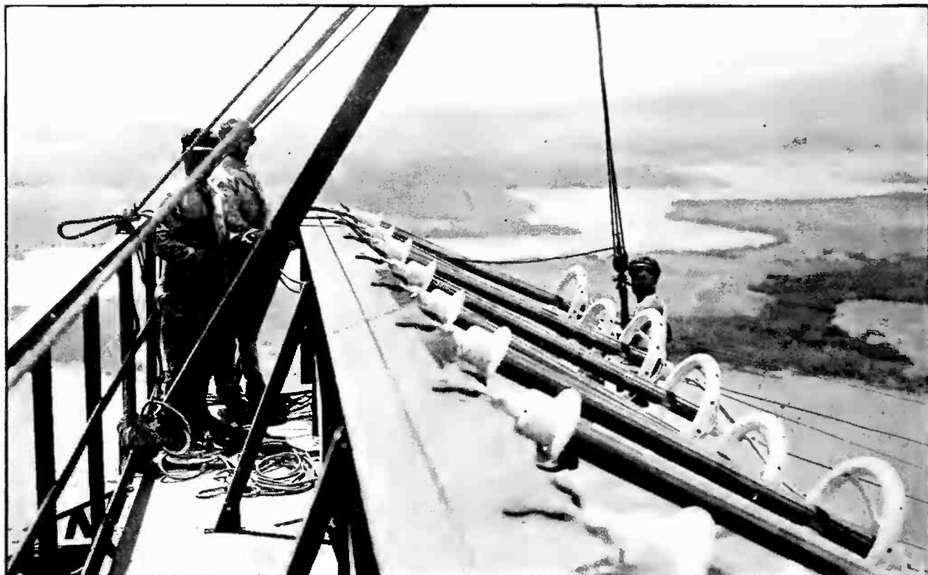
Riggers replacing a defective insulator in the Navy's Pearl Harbor high power radio station antenna
