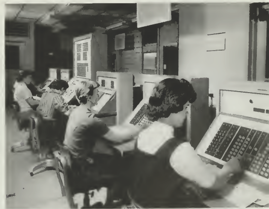
8. All of Bizmac's 220 units can be operated by remote control from this room, known as System Central, which is similar to a telephone exchange.
