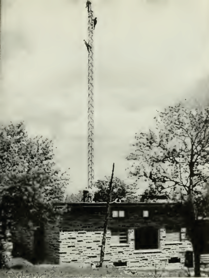
Workmen rig a temporary television antenna atop the transmitter building of CBFT, Montreal.
