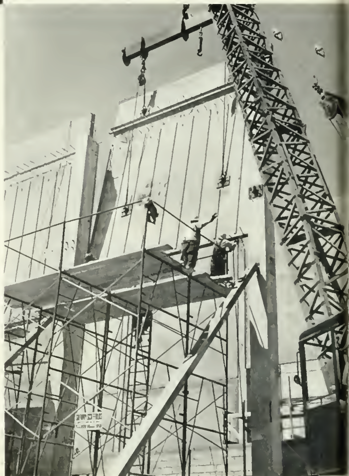
A huge crane swings a 16-ton concrete panel into place as part of the studio's outer wall.
