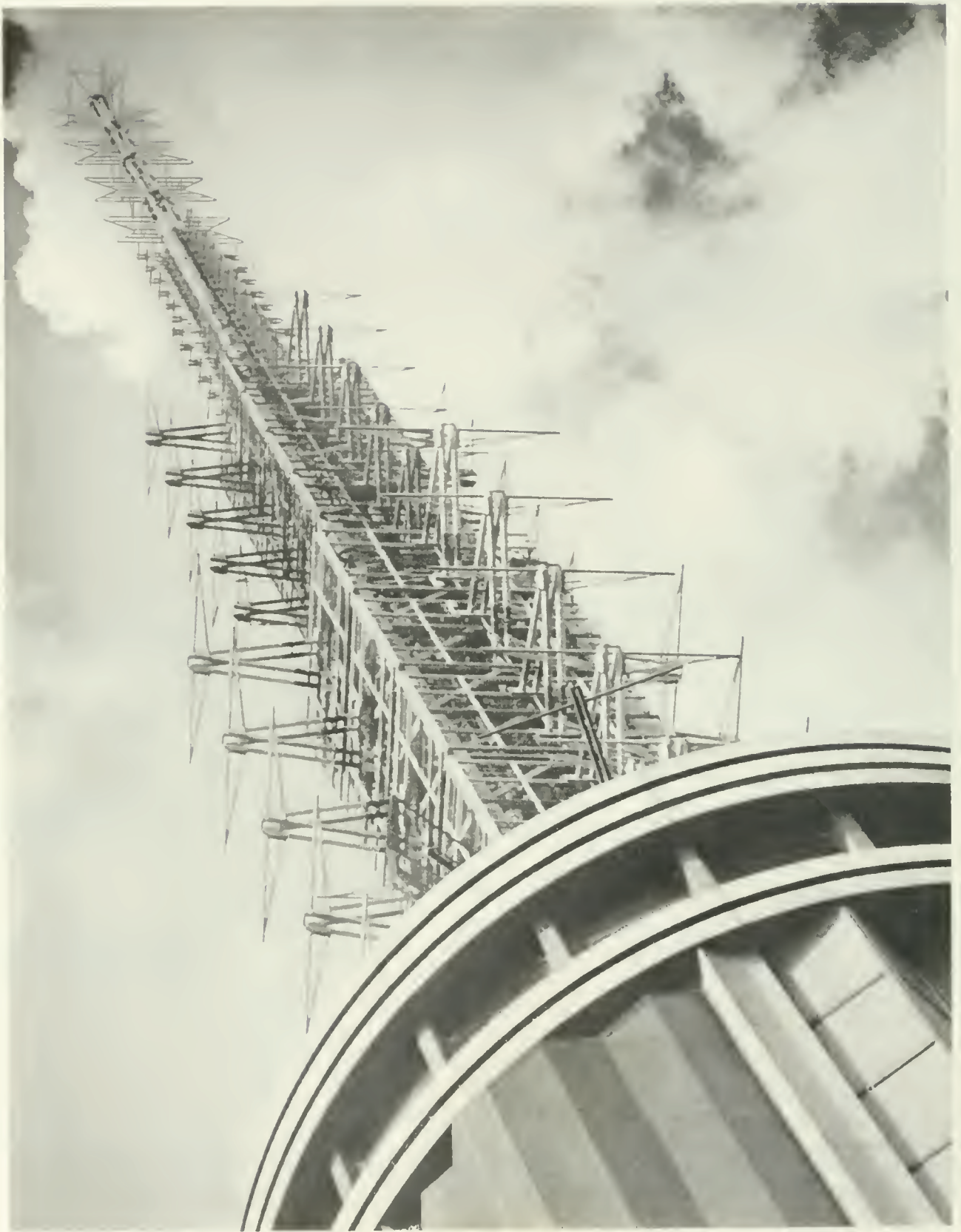
Antennas for five TV and three FM stations are supported by this 200-foot mast atop the Empire State Building. The array was designed by RCA engineers.
