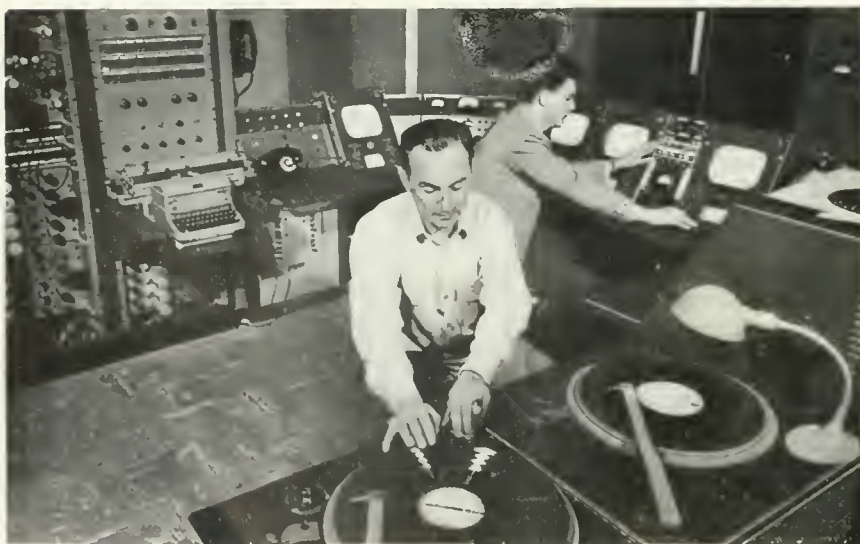
MASTER CONTROL ROOM OF TELEVISION STATION KRON-TV WITH VIDEO MONITORS IN REAR AND TRANSCRIPTION TURNTABLES IN FOREGROUND.
