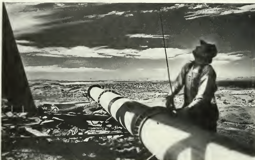
PYLON ANTENNA OF KNBC'S FM STATION ABOUT TO BE LIFTED INTO POSITION ATOP SAN BRUNO MOUNTAIN, HIGHEST POINT ON THE PENINSULA.
