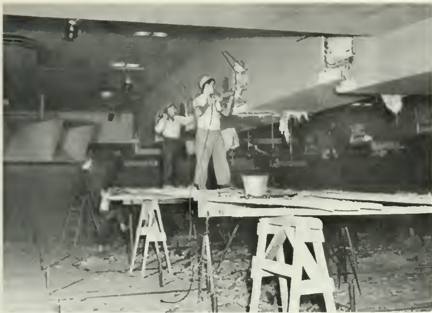
IN REVAMPING NBC'S FAMOUS CONCERT STUDIO 8-II, WORKMEN REMOVE CEILING BEAMS TO MAKE WAY FOR A STEEL OVERHEAD CONSTRUCTION.
