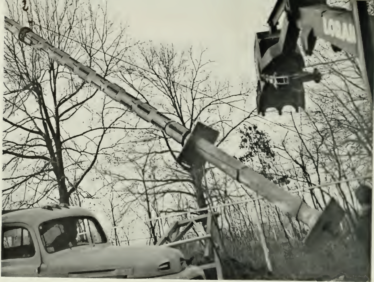
WORKMEN HOIST THE 40-FOOT UHF ANTENNA INTO PLACE AT NBC'S NEW EXPERIMENTAL TELEVISION STATION NEAR BRIDGEPORT, CONN.
