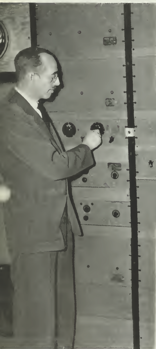
O. B. HANSON AT THE PANEL BOARD OF NBC'S NEW TIME CONTROL SYSTEM.
