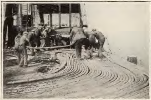
Uncoiling the sea-earth section of the new permalloy cable off Hammels Beach, near Rockaway. The cable weighs from 20 to 36 tons per mile and the men who handle it on the barge must show considerable dexterity to keep it from getting out of hand
