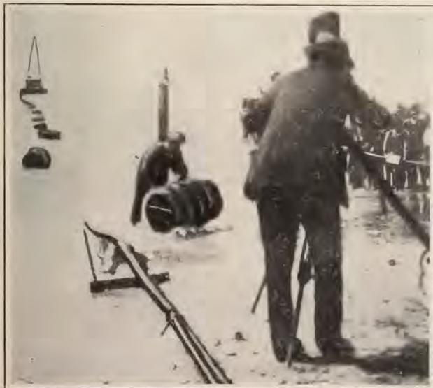
Bringing the shore end of the cable in from the barge by floating it on barrels
