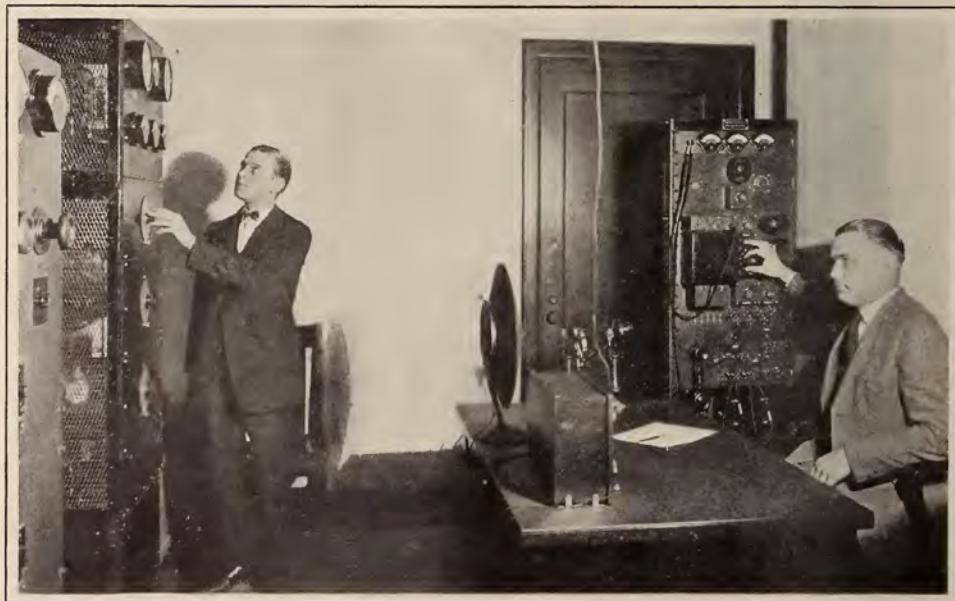
Operator Bennett, at the panel, and Operator Ryan, at desk, of the radiophone transmitter belonging to WHO at Des Moines, Iowa
